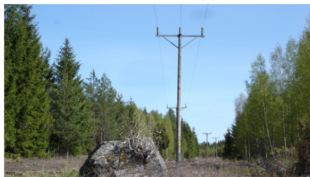
(b) An overhead line, [10]
